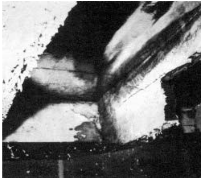
Whether vented or unvented, a wet crawlspace can lead to structural decay.
