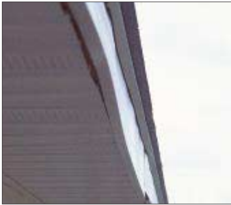
Figure 1. This aluminum fascia, installed in cold temperatures with no allowance for movement, buckled when summer temperatures caused it to expand.
