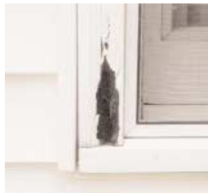
Marvin windows built during the second half of the 1980s have been plagued with rot problems. The window company's lawsuit blaming PPG's preservative was recently thrown out by a federal court.
