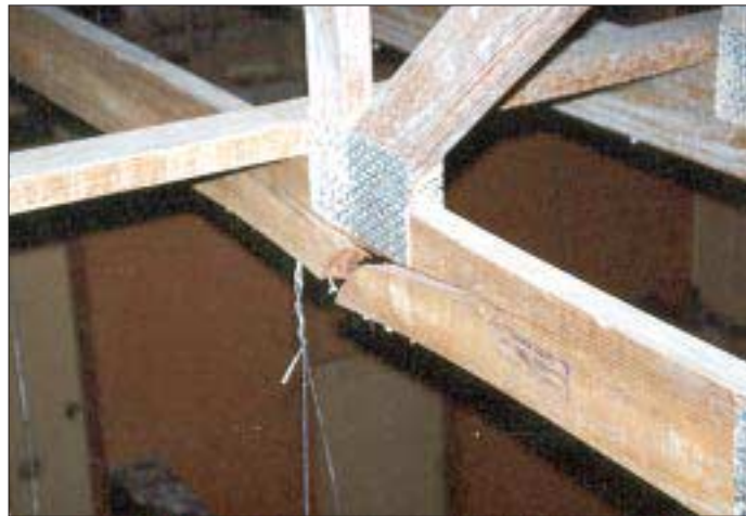
The bottom chord of this FRT truss broke in service. Tension members are especially vulnerable to damage.
