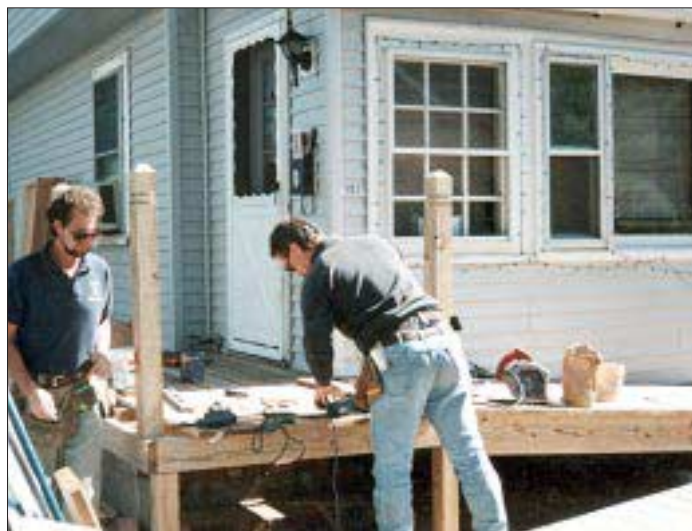
Carpenters with Walden Construction spend a weekend building an access ramp during Rampathon '93.
