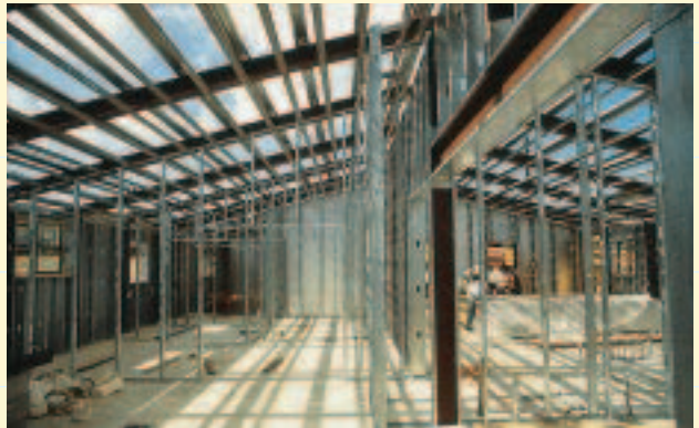
Red-iron framing defines the building’s structure (top), while light-gauge members fill in partitions and skin (above).
