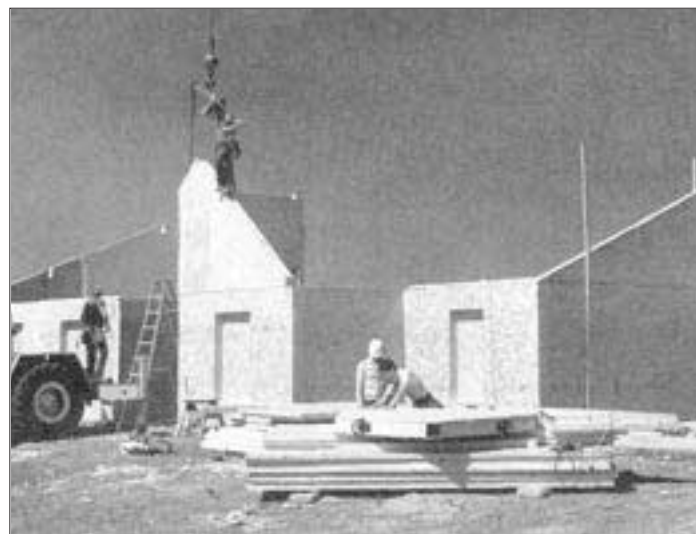
At 400 lbs. apiece, Agriboard's compressed-straw structural panels have to be lifted into place by crane. The company says shell erection takes three to four days.
