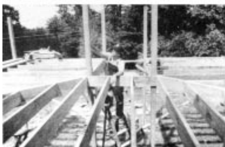
Workers wear neither gloves nor masks to cut borate-treated wood since the treatment is about as safe as table salt. The finished deck frame (inset) takes shape on a N.H. home.
