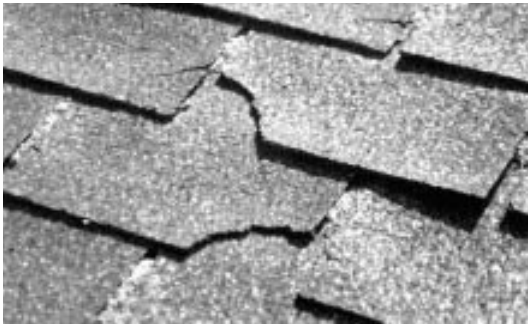
Roofers say tears and granule loss are destroying many 20-year shingles well before their warranties expire.
