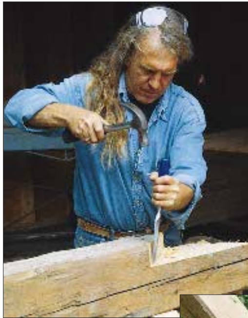
A carpenter crafts a joint for one of four timber trusses that will support the roof of the addition.
