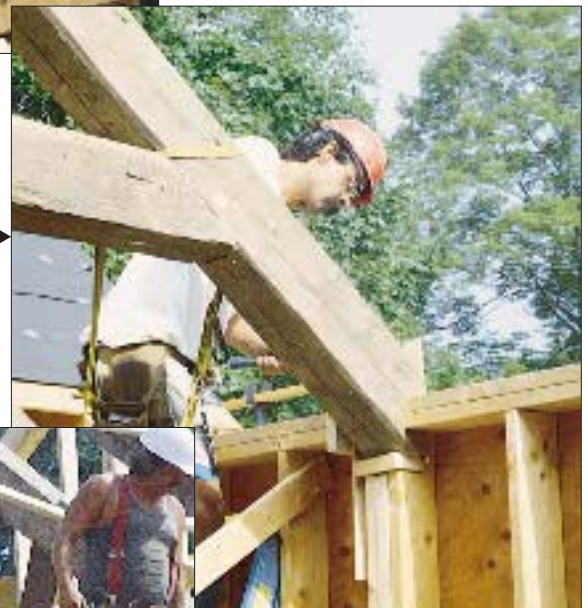
The crew used a crane to hoist the trusses into place on top of built-up posts in the stick-framed wall.
