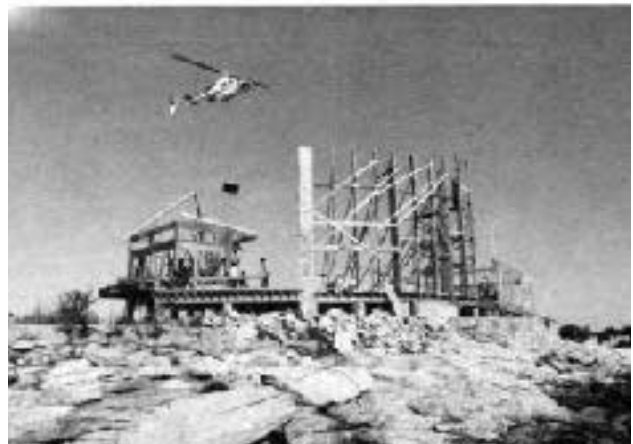
The helicopter completed its task of shuttling materials and hoisting beams into place in the course of just one day. Here it is about to set down a cargo-net-load of plywood on the landing area nearby the house.
