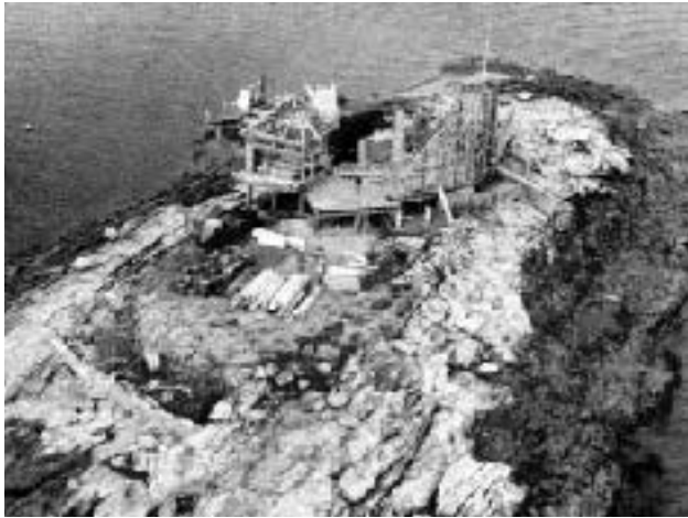
Most of the materials needed to build this 2,800-square-foot house, situated 1/4 mile off the coast of Connecticut, were brought to the island by helicopter.
