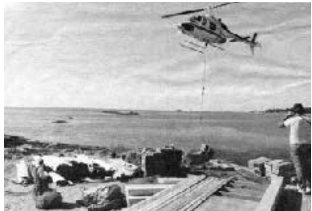
Considering the cost of getting a crane to the island, and the cost of double handling all the materials for the project if they were shipped out on barges, the helicopter, shown here lifting a cargo net full of shingles, was an economical choice.
