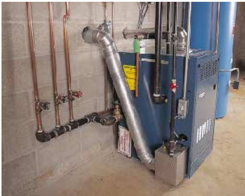
Figure 2. A galvanized pipe (foreground) provides combustion air directly from the exterior to the burner of this sealed-combustion boiler. A separate galvanized vent pipe conducts the flue gas through the sidewall.
