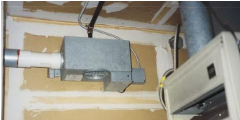
Figure 7. A forced combustion air system uses a fan to introduce makeup air into a utility room. This permits the use of a much smaller duct than when the makeup air enters by gravity.
