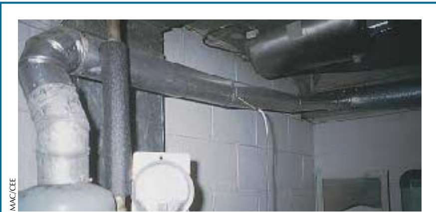
Figure 1. Avoid long horizontal runs of vent pipe, which can cool the flue gas and reduce the draft. This gas-fired water heater should have been located closer to the chimney.
