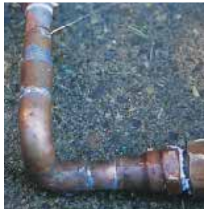
This photo shows a section of copper tubing removed from an elderly housing project in Lyndonville, Vt. A series of pinhole leaks caused damage to interior finishes.
