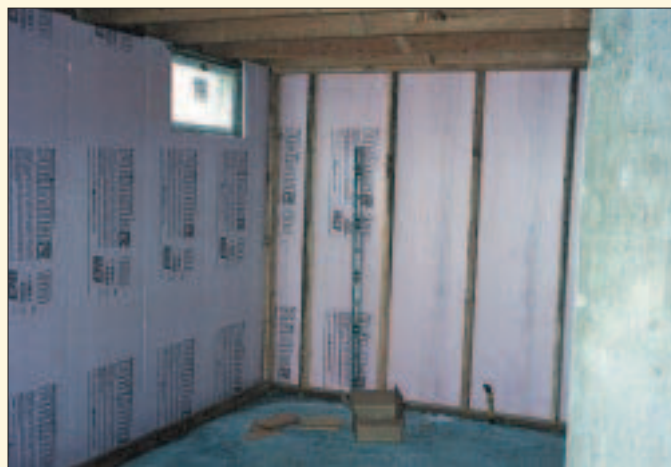
Figure 3. The author glued foam insulation to the basement walls, and added an insulated 2x4 wall within that.
