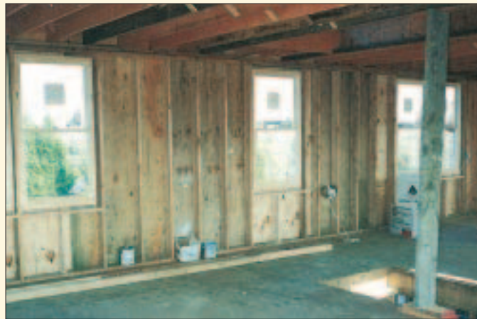
Figure 2. A load-bearing double band joist allowed the author to eliminate headers and double jacks from his exterior walls. The 1 1/2-inch space between the windows and the framing around them was easily filled with spray cellulose.
