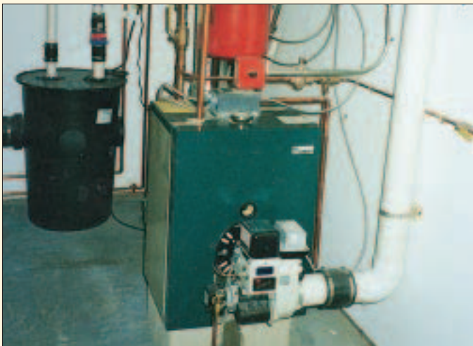
Figure 6. A dedicated PVC duct in the basement brings combustion air directly to the boiler.
