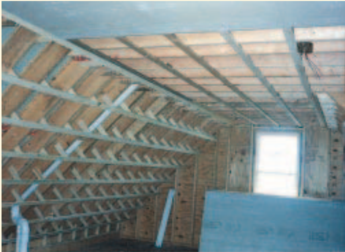
Figure 4. Building down the attic ceiling with strapping made plenty of room for blown insulation, without the expense of oversized rafters.
