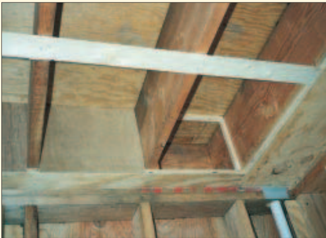
Figure 5. The author paid special attention to band joist areas, boxing out each cavity with plywood and filling it with blown cellulose.
