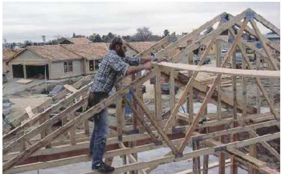
Figure 4. A carpenter nails off the top chord brace at the premarked layout line, automatically spacing the trusses. Note in the background how the outriggers have been installed in preparation for the barge rafters.
