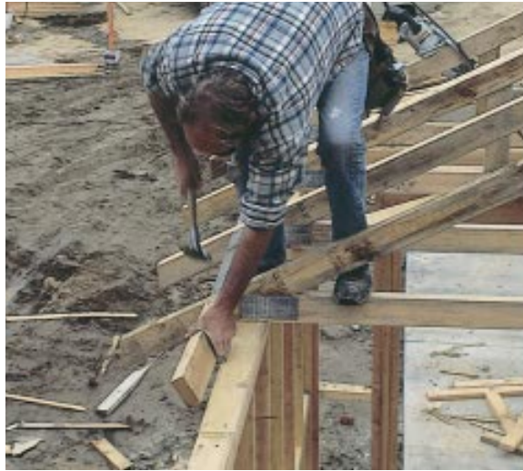
Figure 5. With the efficiency that comes from good preparation, an eaves block is installed (right), then the next truss is rolled up and nailed off (below).
