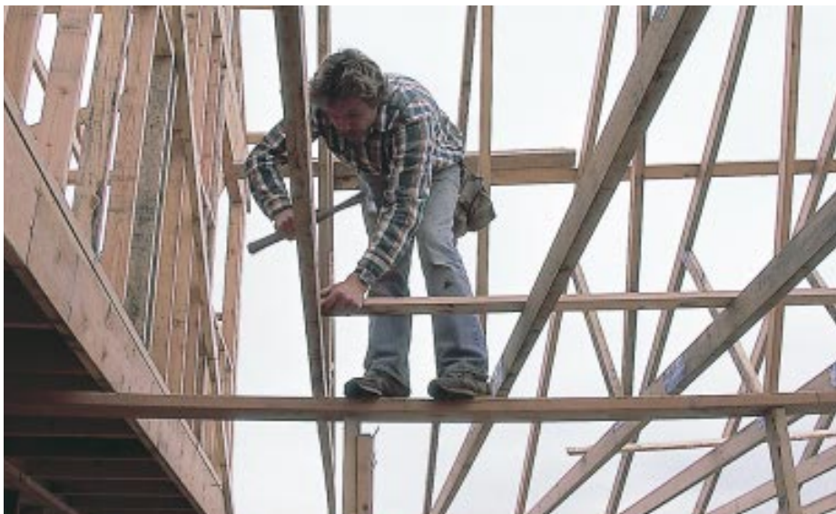
Figure 6. Permanent bracing, which the author calls lacing, is installed at specific locations identified in plans from the truss manufacturer.
