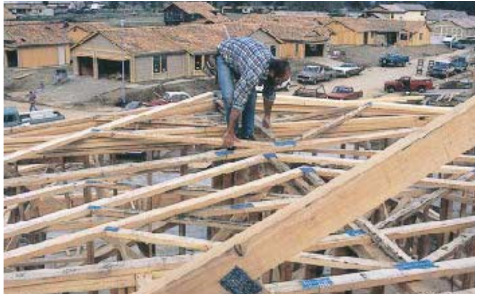
Figure 3. Unless trusses are too big to handle twice, spreading out trusses along the top plate makes it easy to roll them up into position later.
