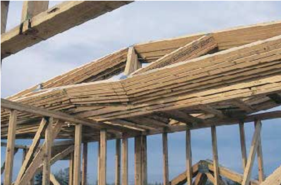
Figure 1. Small trusses (under 30 feet) can be spread evenly along the walls. The author prefers to stack larger trusses in bundles, so he only has to move them once.
