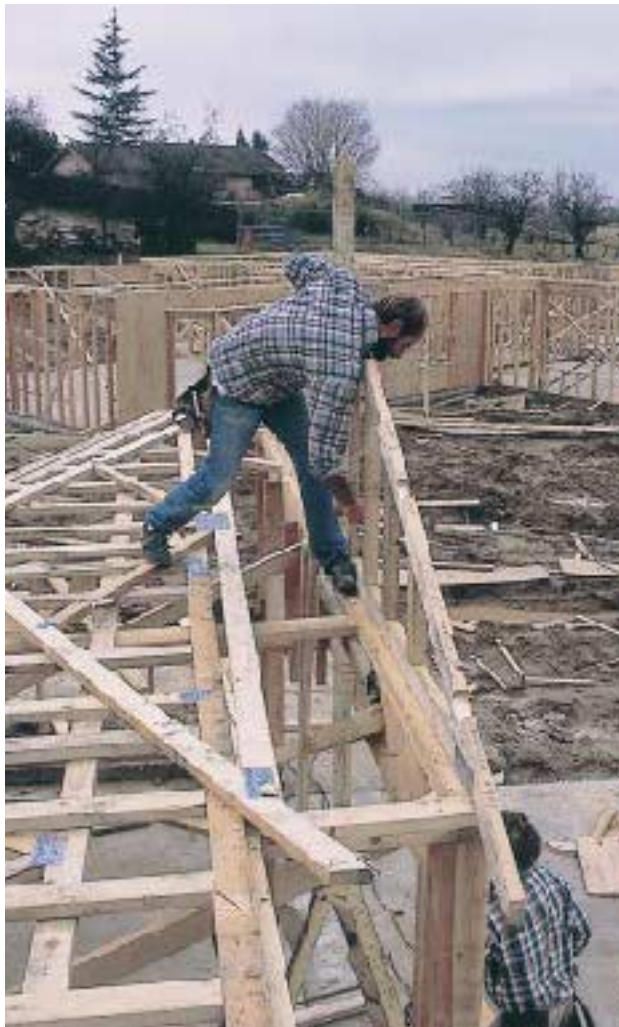
Figure 2. With the upright braces in position and toenails started along its bottom chord, an end truss is tipped into position and nailed off. On taller trusses, the author preinstalls the top outriggers to avoid later hassle.
