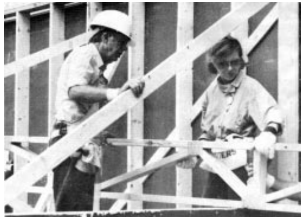
With Carter's help, a Charlotte, North Carolina Habitat for Humanity project completed 14 houses in just five days.
