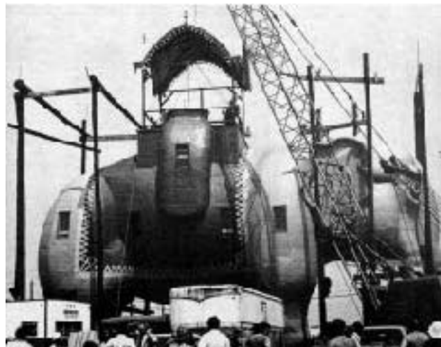
Lucy the Elephant undergoes finishing touches on her "howdah" or observation deck. She was moved to this Margate, N.J. city park in 1970. No, she was not packed up in a trunk. Instead, she was cribbed and trucked on I-beam supports.
