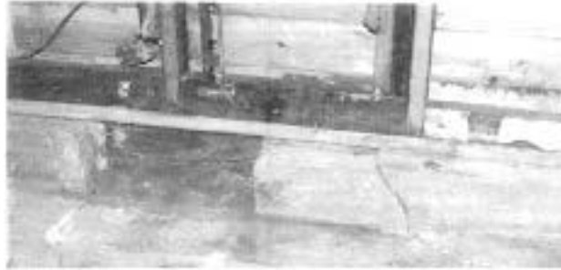
Cracked foundation linked to frost heave. Recommendation: Before repairing, improve the drainage.
