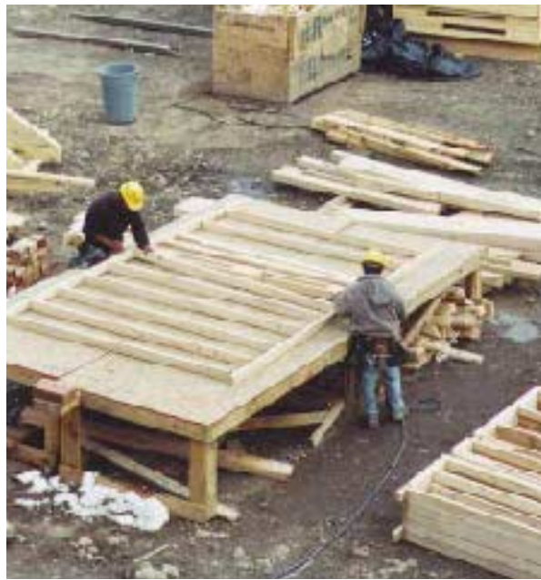
Figure 6. Carpenters assemble pre-cut wall panels on site (left). Wall plates are stacked at the far end of the table, headers, sills, cripples, and tees are stacked to the left, with finished walls to the right. Everything required is in the package. The compact lumber packages will result in an enormous pile of wall panels. Two short walls at the bottom of the pallet are used to create clearance for the forklift (below). Carpenters can spread and erect wall panels very quickly. Notice how clean the area is (bottom).
