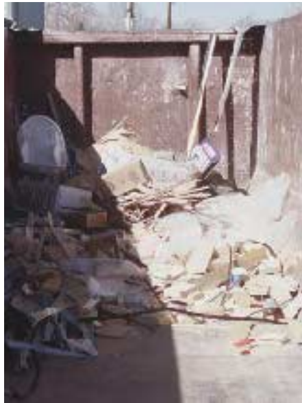
Figure 7. This is all of the framing waste from a 60,000-square-foot project, plus somebody else's trash — barely a small pickup load.
