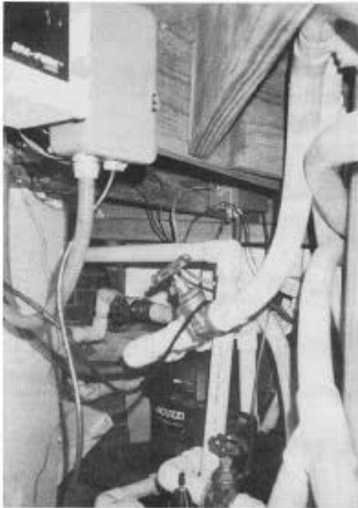
They weren't thinking about the electrician (or the plumber) when they buried this hot-tub motor and pump under a deck set 18 inches off the ground—says the author, who faced this mess on a recent job.
