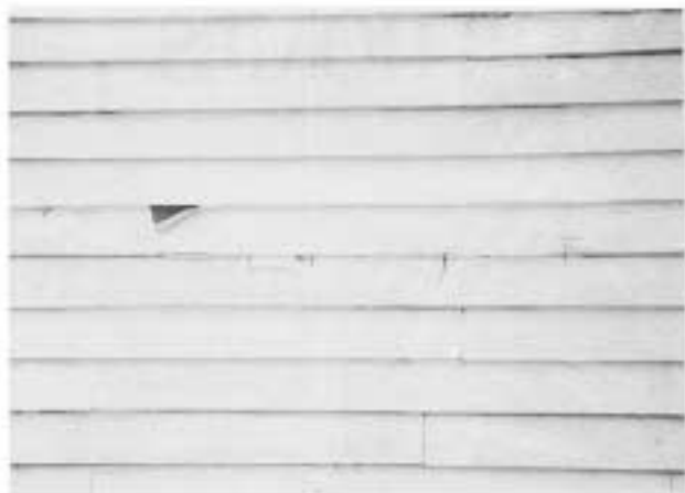
Make sure you prep and paint the butt edges and butt joints—to prevent this type of water penetration and peeling. Also avoid painting when the wood is swollen with moisture—lest it shrink and crack the paint at joints. This is more common with oil-base paint, since it's less flexible than latex.
