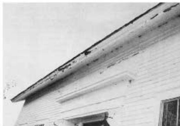
Backed-up water from ice dams can wreck both interior and exterior finishes—including paint on soffits, fascia, and siding.
