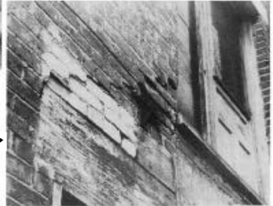
The star anchor is safely secured to the wooden floor structure. Unfortunately, the brickwork is crumbling around the star—making for a precarious situation
