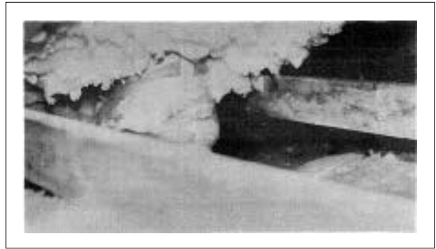
A bath exhaust that vents or leaks into the attic can cause frosty sheathing. When the frost melts, you can get moldy wood or wet ceilings.
