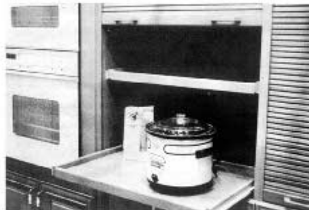
A pull-out shelf for small appliances is mounted here with other 24-inch deep cabinets. It is wired with dual outlets in back of cabinet, and has a tambour door.
