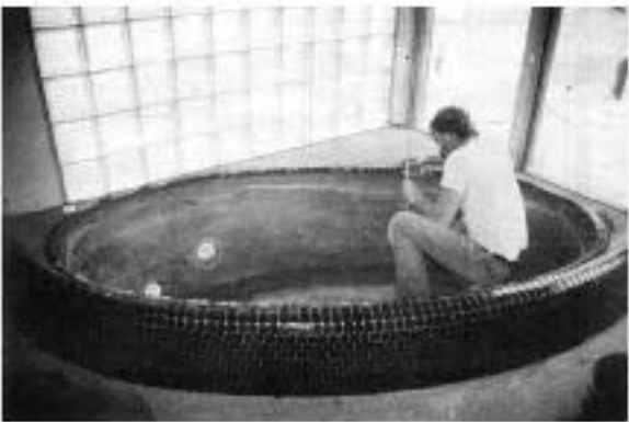
(1) The sunken tub starts with a braced plywood form on a concrete-slab base. Patches of CPE membrane are sealed to the jets with butyl caulk where they enter the tub. (2) Pieces of membrane cover the entire tub surface and all seams are lapped and sealed with butyl. (3) Galvanized metal lath is attached to a steel armature (9-gauge gal. wire) inside the tub. (4) The tub gets a heavy mortar bed and tiles are finally thin-set to the mortar bed.
