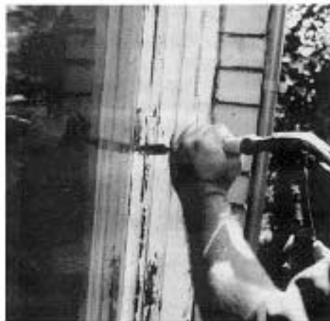
Chiseling out the old putty. Smack the putty in the middle to break it in half. Most of the stuff will just jump out.
