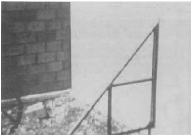
Don't backfill a block wall unless the floor joists are in or the walls are securely braced with temporary supports.
