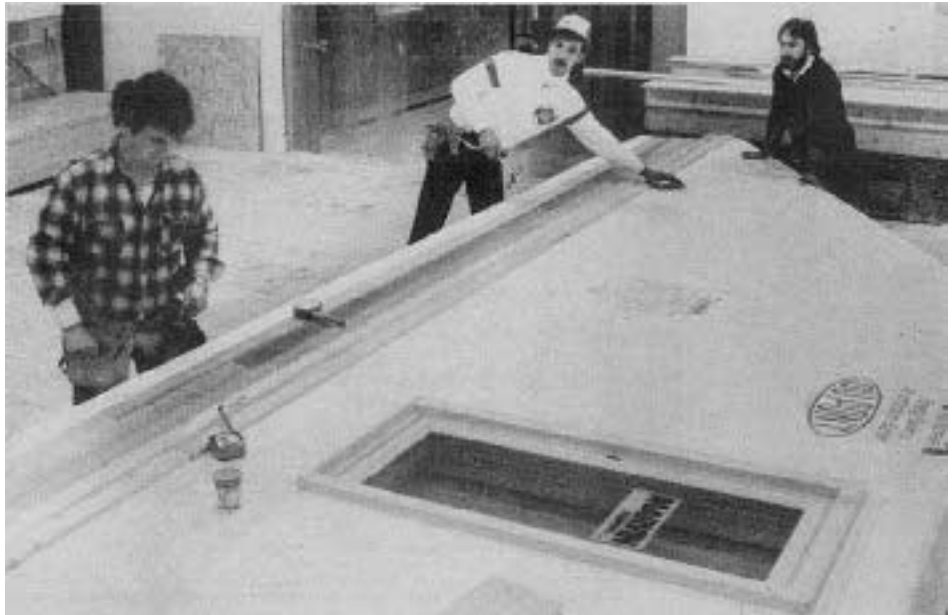
Three ABS employees construct a building module which contains a Marvin window and Tyvek. Most of the materials ABS uses in building its components are standard U.S. fare, although it does import gaskets and vapor barrier material from Sweden.
