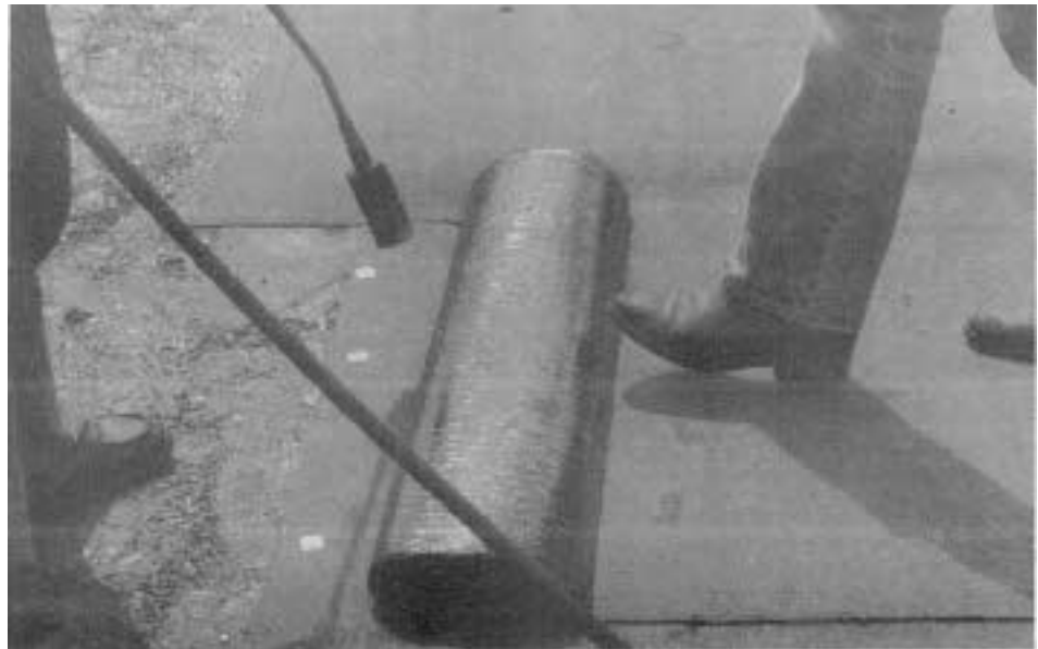
Applying modified bitumen with a hand-held torch demands care and safety precautions. The applicator must heat the membrane until it just turns shiny but before it begins to run.
