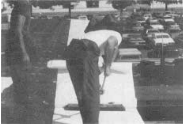
A worker uses a flat broom to force down the self-adhering membrane to get a good bond to the substrate.
