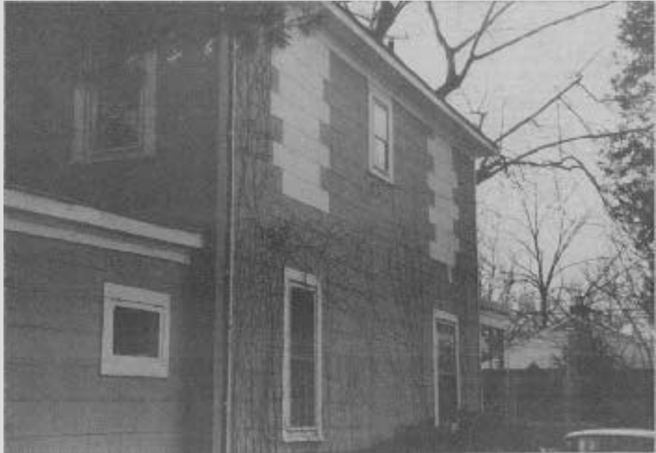
This 1920 frame house had two of its 23 windows removed to avoid expensive repair.
