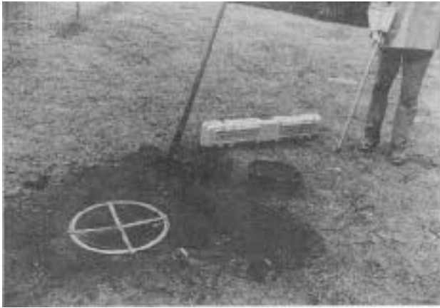
High-tech comes to the rescue. The hand-held wand can locate a small transmitting "mole" attached to the end of a snake. Here the snake is inserted through the tank outlet to locate the leach field or drywell.
