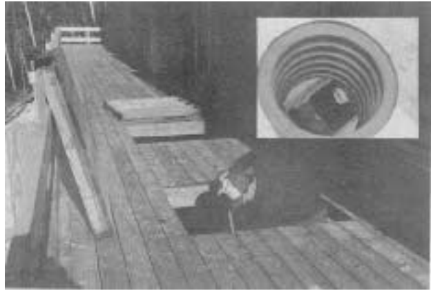
Ideally, septic tanks will have inspection hatches at both the inlet and outlet. Here, hatches in the deck allow access to the lids. And plastic culvert pipes (inset) form lid extensions from the ground surface to the tank.
