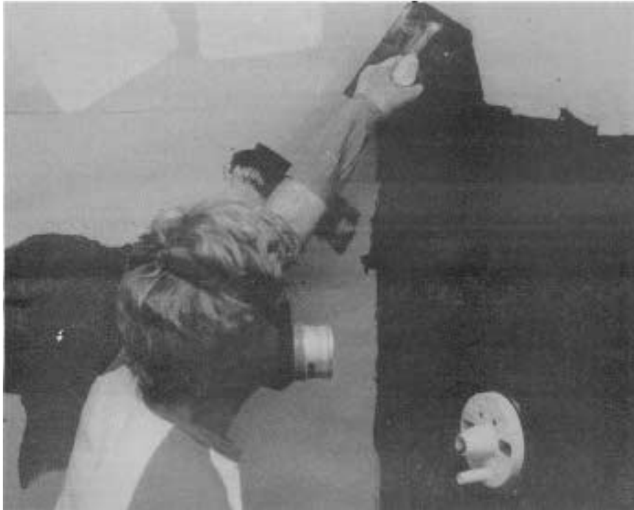
Figure 1. On a tub enclosure, the author coats the water-resistant drywall with cold-patch asphalt, then with tar paper. Next goes metal lath, a mortar bed, and finally - the tile.
