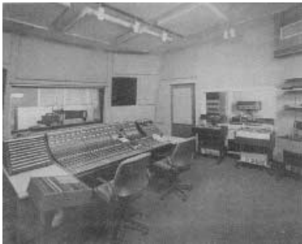
Operators at the control console look through the double window into the recording studio. Note sound diffusers on the ceiling and absorber panels on the wall.
