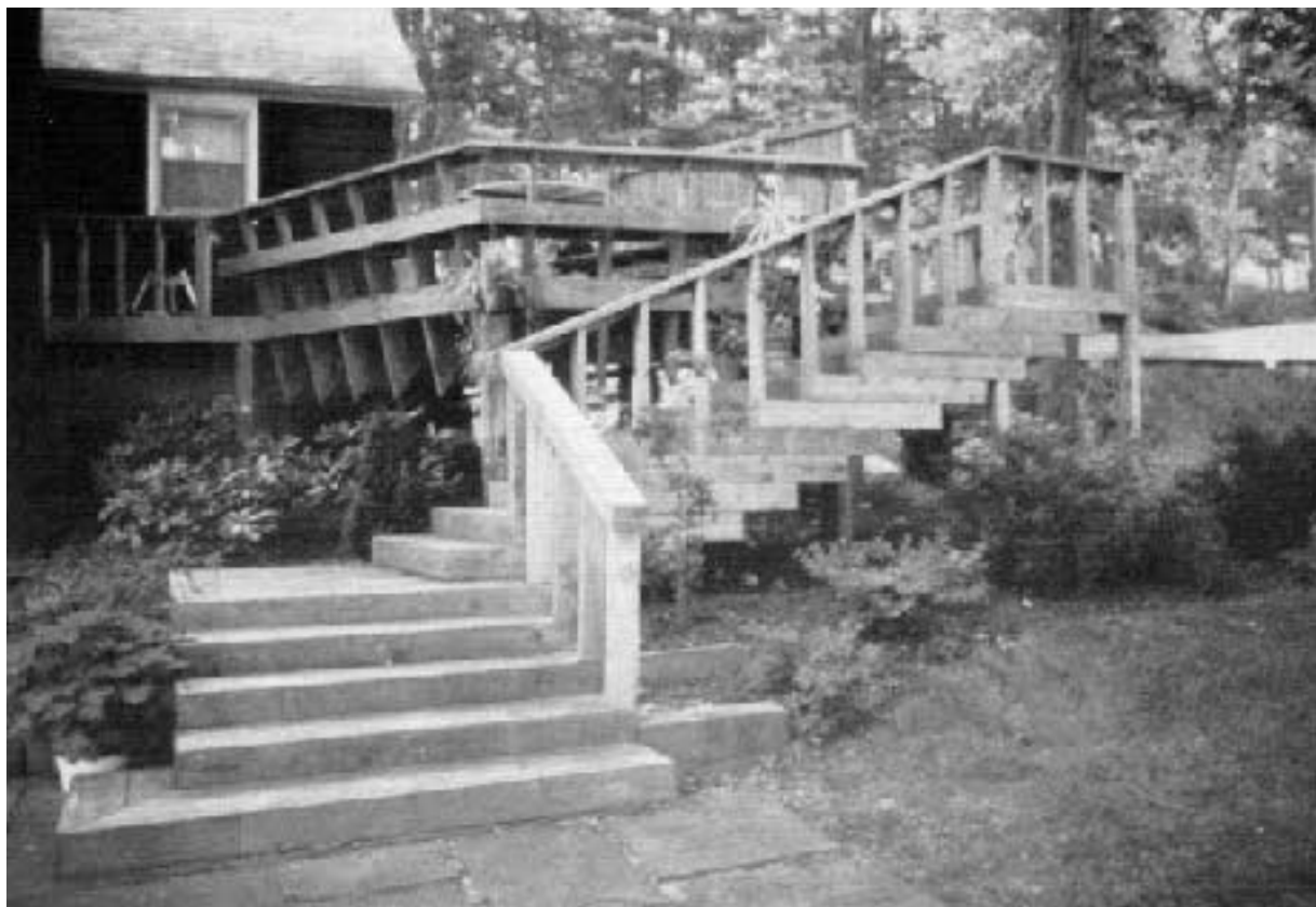
The 2x6 riser returns give the appearance of terraced stairs. Also, note how the angled railing posts and bench supports are extended downward as a design element.
