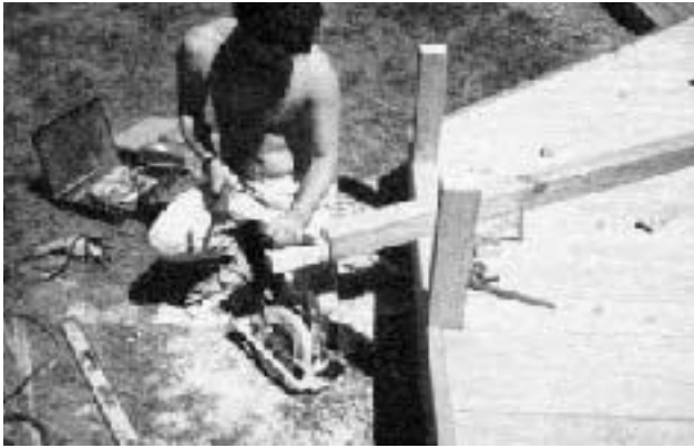
Figure 8. Attach a post by notching it through the decking and bolt it to the joist from the inside. The post can be flush with the outside perimeter joist.
