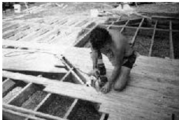
Figure 6. Decking boards can be left long and trimmed all at once. Here decking will change directions, with a trim piece marking the joint.
