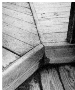
Figure 7. A perimeter-rim joist covers deck-board end grain and cleans up the look of the deck. Note the dividing board on the seam in the deck.
