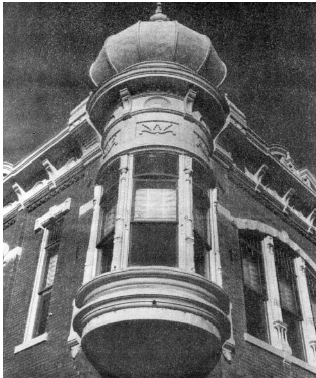
Figure 4. Don't ruin a historic facade when you replace windows. The tower should have had a curved glass window installed. But the replacement windows on the side facade look okay.
