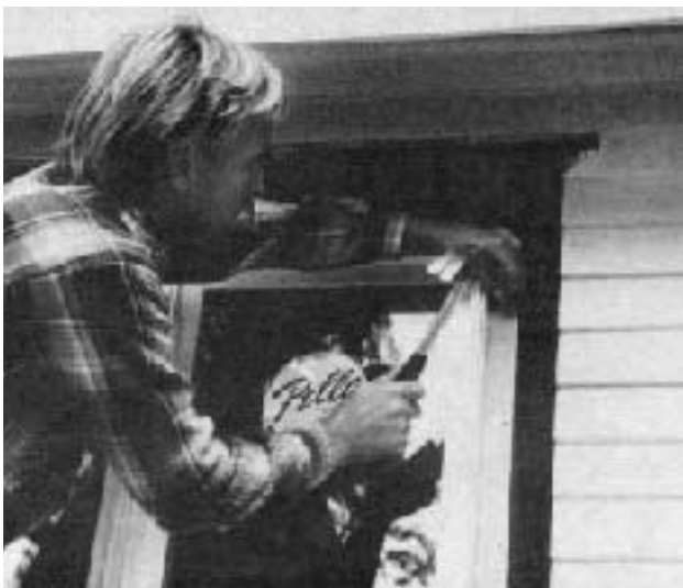
Figure 1. These windows were custom-made to fit the rough opening. They required the removal of the exterior and interior trim.
