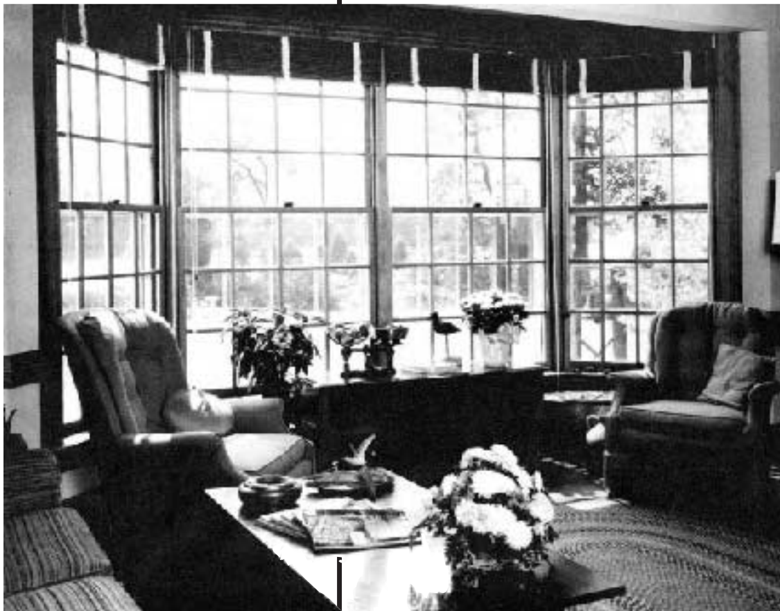
These replacement windows, made of wood, duplicate the original muntin arrangement and were stained to match the existing woodwork.
