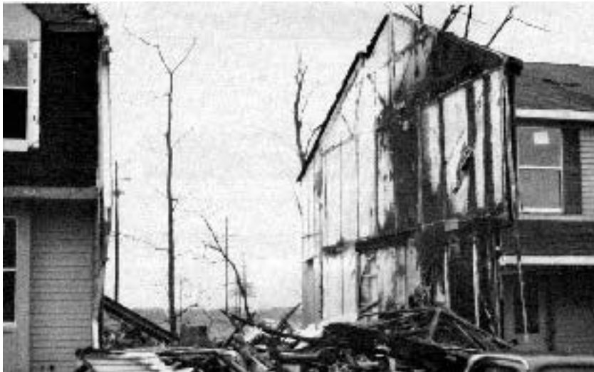
There's a good reason party walls are also called firewalls. Two-hour gypsum-based firewalls prevented this townhouse fire from spreading; break-away features in the framing allowed the structural framing that burned to collapse and fall away from the adjacent units.
