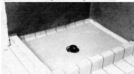
A careful cut in this PVC membrane exposes the lower part of the drain assembly, allowing the upper flange to be bolted on. The completed pan (inset) is ready for mortar bed and tile.
