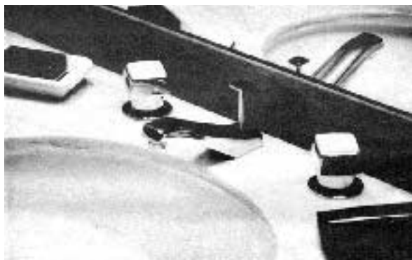
Figure 3. Kitchen, bath, and bar sinks are all specced with Faucets that have 2.0 gpm aerators. As these are lost or removed, they are replaced with a tamper-proof model.
