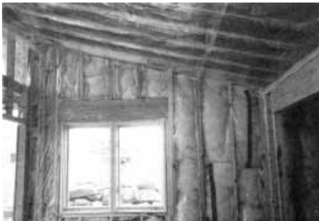
Vapor barriers are a key part of the defense against moisture problems. Seal the joints and penetrations as well as you can within reason.
