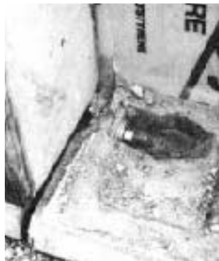
Figure 1. Installers join Superior Walls panels with bolts at the top and bottom. A cast-in "bolting saddle" reinforces the joint.
