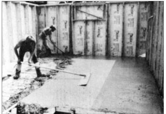
Figure 4. After setting the panels in place, it's time to pour the slab. Note the cast-in-place concrete studs with wood nailers on their interior faces.
