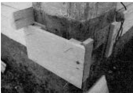
Figure 2. Cut all pieces of trim to fit and nail them in just enough for placement. Then, remove them with nails still in place, and prime.
