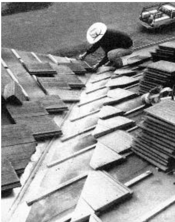
Laying out and snapping a single line for valley cuts ensures a crisp looking closed valley and the chance to do the cutting all at once. The tiles on the right have already been cut and set aside.
