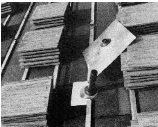
Figure 3. This base flashing or "subjack" at the vent stack will be covered by tile and then by the top flashing that is sitting next to it. This kind of care helps the roofing system last as long as the tile itself.
