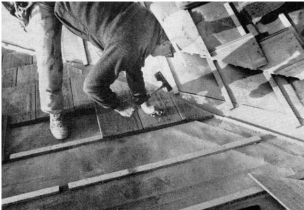
Figure 6. Nailing tiles within 36 inches of a valley (without nailing into the valley metal) is required even on low slopes where field tiles aren't nailed. The 7d galvanized nails are driven just one tap short of snug to keep tiles from breaking and to give them a little room to move.
