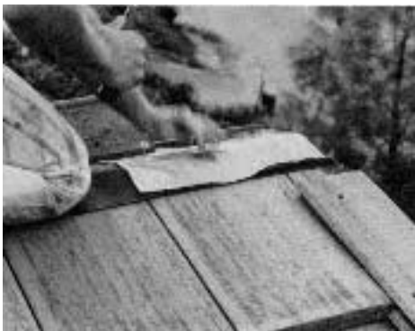
Figure 7. After forming and fastening a lead flashing at the ridge (top), the author miters the rake tiles at the peak, and installs them along with the first ridge tile (bottom). Successive ridge tiles are daubed with mastic where they lap.
