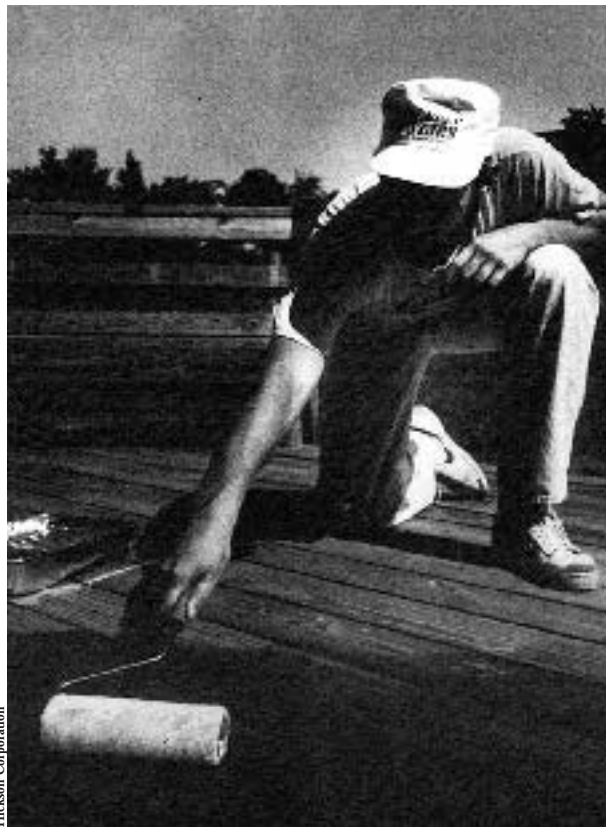
A painter rolls on a water-repellent coating to protect the pressure-treated decking from weathering.
