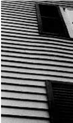
Figure 1. This hardboard has absorbed excessive moisture and expanded, causing buckling and bowing. Note how tight and swollen the butted joints are.
