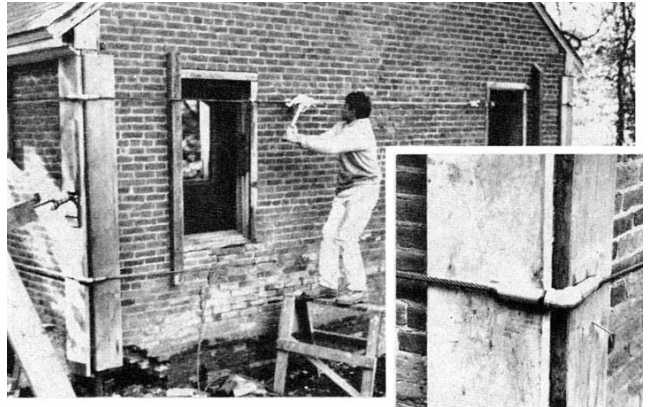
Figure 2. To draw the cracks together, cables were wrapped around the house and drawn tight with come-alongs while the fallen corner was jacked up. An additional jack, braced at a diagonal, helped push the structure back in place. Note the cable runners made of steel pipe (inset) to prevent the cables from binding on the corners.
