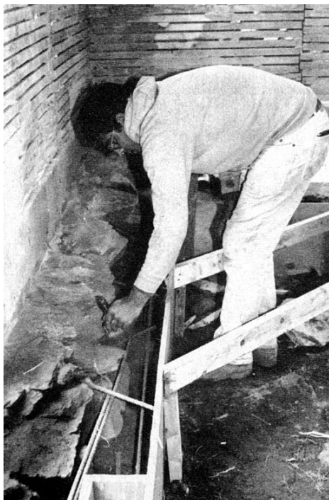
Figure 3. The old fieldstones were dusted off and then wetted to ensure a tight bond with the concrete. Note the pocket built into the foundation in the foreground of the photo for a midspan joist beam.
