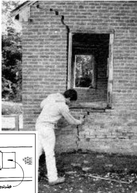
Figure 1. Stepped cracks opened up at the window corners when one corner of the building settled. The inset illustrates how the wall pivoted outwards when the fieldstone foundation sagged.
