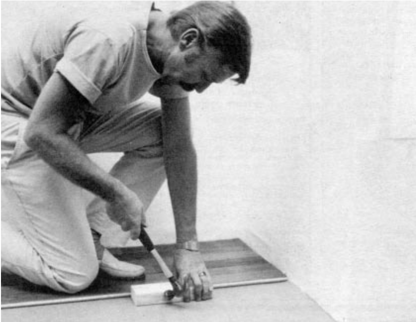
A worker installs a long-strip floor panel over a linoleum floor and uses a 2x4 block to set it in place.
