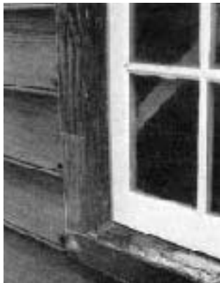
Figure 1. Wood dutchmen were used to repair rotten small areas of muntin and the bottom corner of the frame. The new window sill was milled to the same profile as the original because it was too deteriorated to repair.
