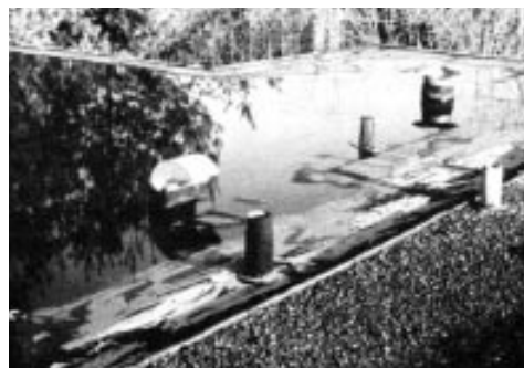
Most roofing — and material warranties — will not stand up to ponding caused by too little roof slope and poorly placed drains.
