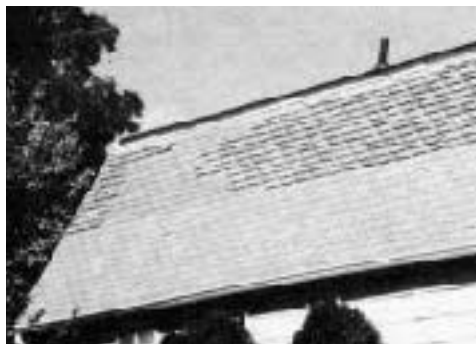
Poor attic ventilation leads to curled shingles in summer (left) and ice dams in winter (below left).
