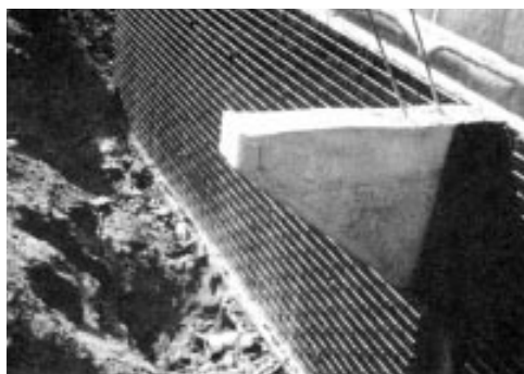
Poured haunches like these (left) allow concrete stoops to sink and rotate (below left).
