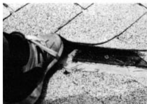
Top corner of shingle in an open valley that wasn't clipped to prevent water penetration, but was nailed through the flashing.
