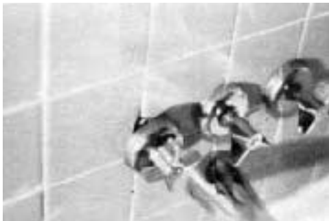
Escutcheons that aren't caulked tight leave an easy path for water to enter walls (left). A grout joint between tub rim and the first course of tiles guarantees failure (below left).
