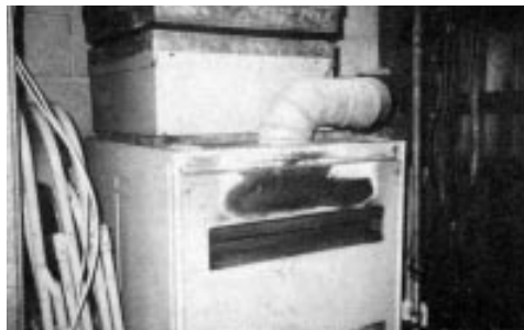
Backdrafting scorch marks discolor the draft hood of a forced-air furnace.
