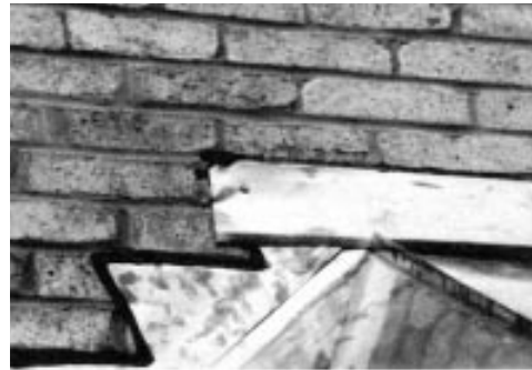
Sidewall flashing cemented to masonry with mastic will last only a few years before pulling away.
