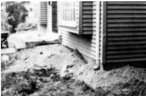
Fill dirt used for corrective grading around foundation where original backfill settled.
