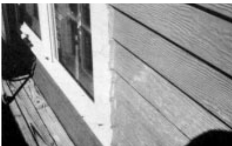
Buildup of caulk where siding dies into window jamb.
