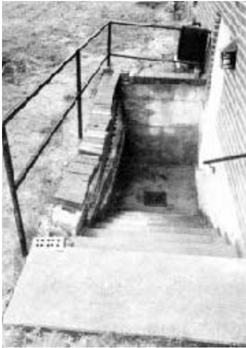
Basement entryway retaining wall buckled by lack of rebar and drainage.
