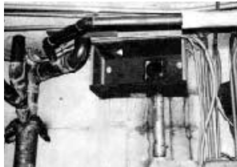
Top-mounted conduit on this electrical box also served as a channel for water.
