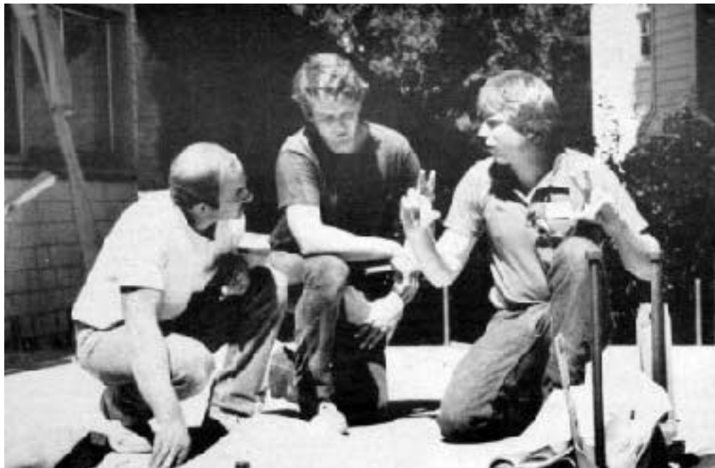
Project manager Farrell, at right, reviews the coming week of framing with his carpenters, and coordinates the start dates for his subs.
