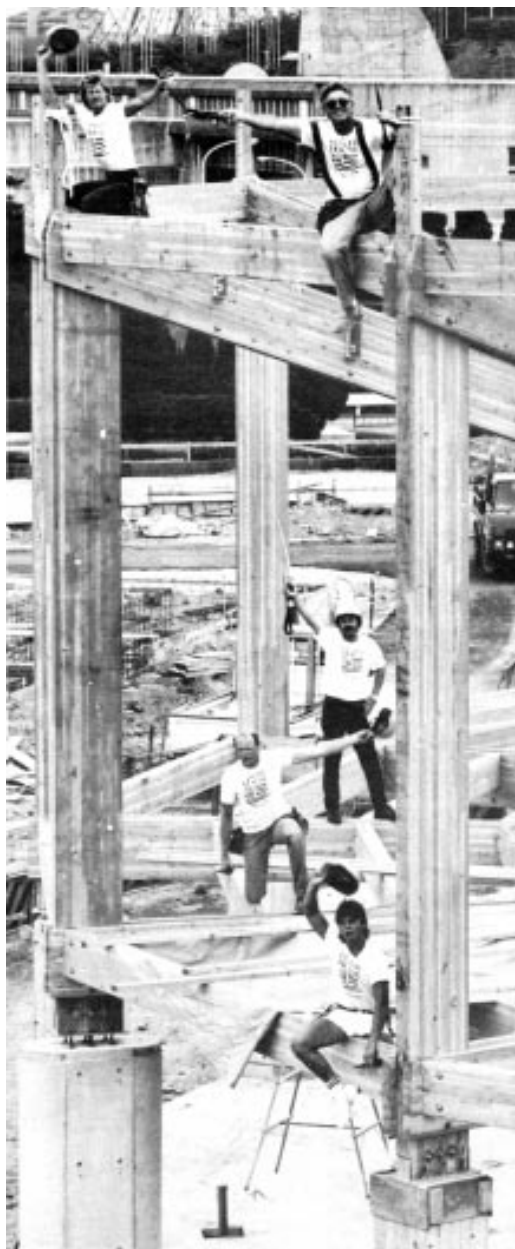
American and Japanese carpenters worked together to build the doughnut-shaped "Supermarket of Homes" in Osaka. The structure was built with American-made glulam posts and beams.
