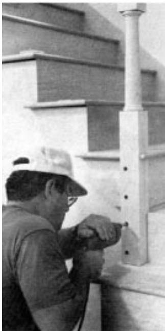
Figure 8. The author mounts the landing newel with either drywall screws or hex-head bolts, making sure that he hits a stringer or framing member with each screw.
